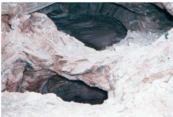
Figure 6. Collapsed horizontal pillar in the mixed salt mining field.
