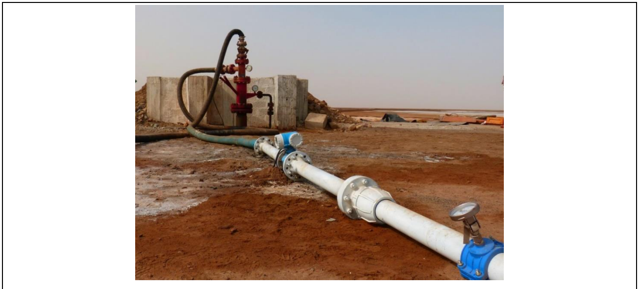
Picture 3: Well head of the test well SolMin01, in the foreground the monitoring devices on the brine line.
