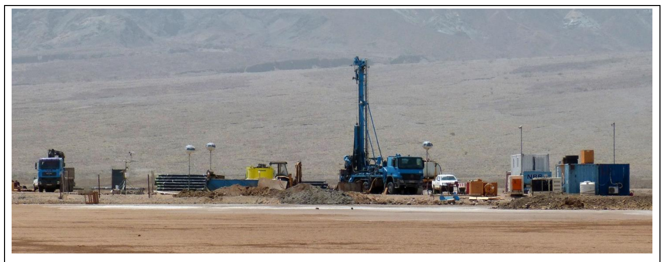
Picture 2: Drill pad during well cementation of the final 9-5/8" casing, drill rig Nordmayer DSB 3-14 of the Company Nord Bohr- und Brunnenbau.
